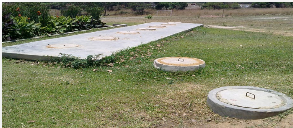
Figure 5. Anaerobic Baffled Reactor (ABR) and Anaerobic Up-flow Filter (AUF)
